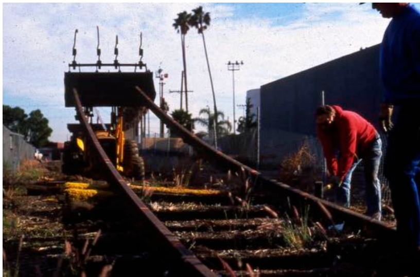
Fig 27: Workmen inadvertently rip up Sleepers/Ties I . Photo. B.,Ely, 1994.
